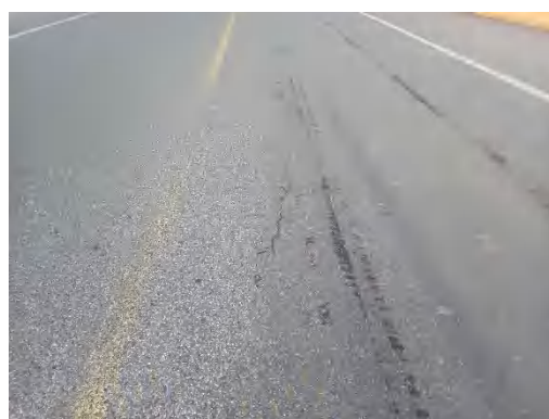
桥面纵向裂缝
